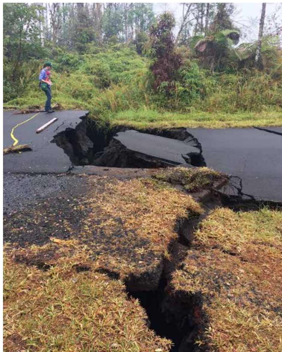
Hawaiian Volcano Observatory geologist stands next to cracks on Nohea Street in Leilani Estates. Prolonged volcanic activity beneath the surface has expanded cracks in the ground throughout Kīlauea’s East Rift Zone. Source: USGS
